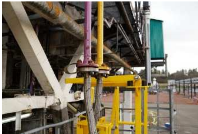
Photo 4 Flexibles coté installation
